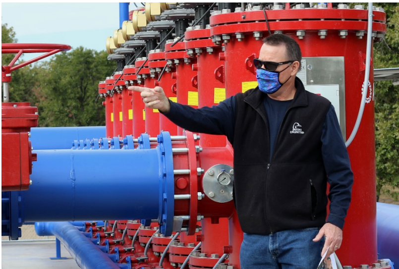
Tim Campbell, Project Manager, FICO, explains the filtration system of the FCAP waterline system.
