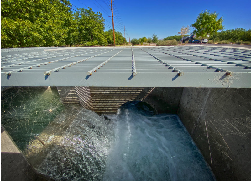
The pipeline system travels underneath an interstate, two railroad crossings, and several other roads and obstacles.
